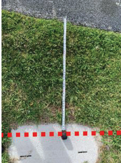
Existing Communication Pullbox
