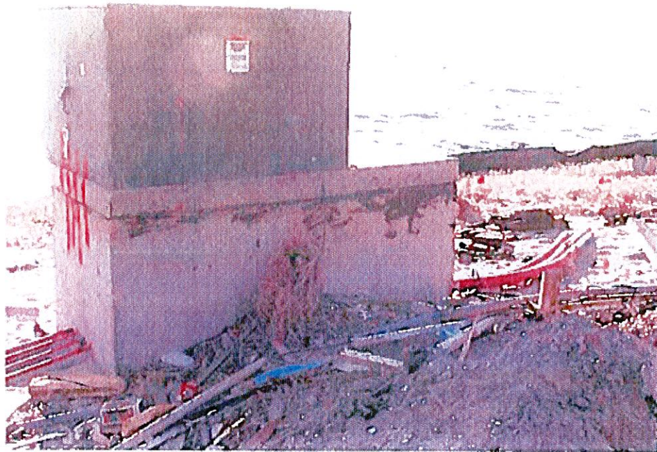
Figure 8-4. Storm Surge Erosion Exposes Underground Cables
