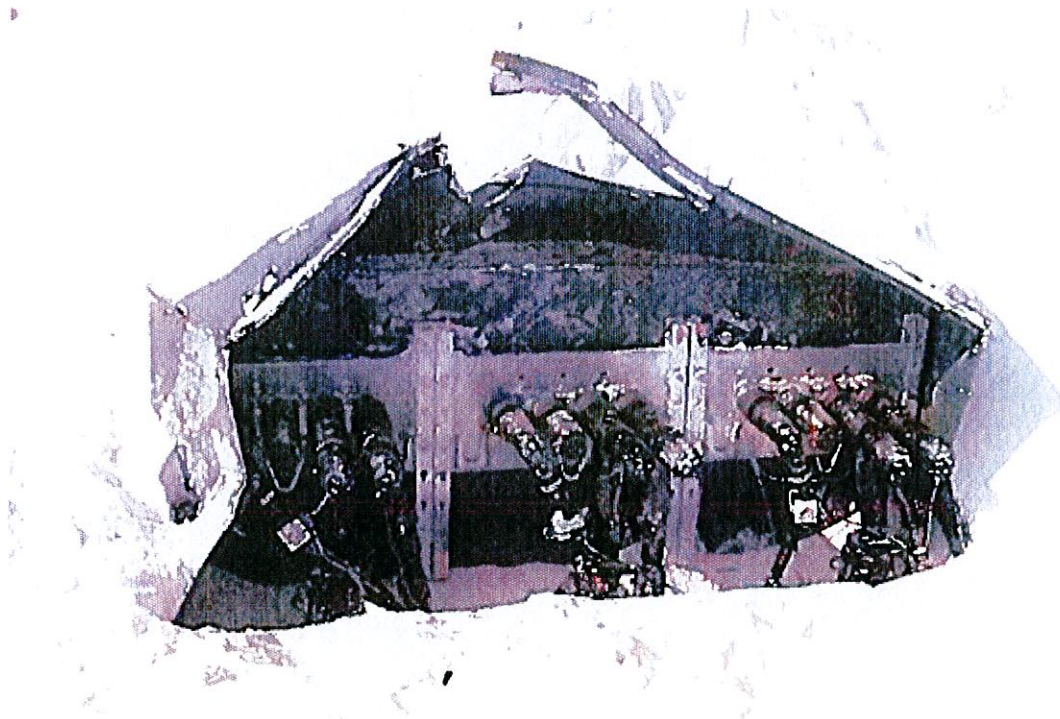
Figure 8-3. Storm Surge Buries Pad Mounded Equipment in Sand
