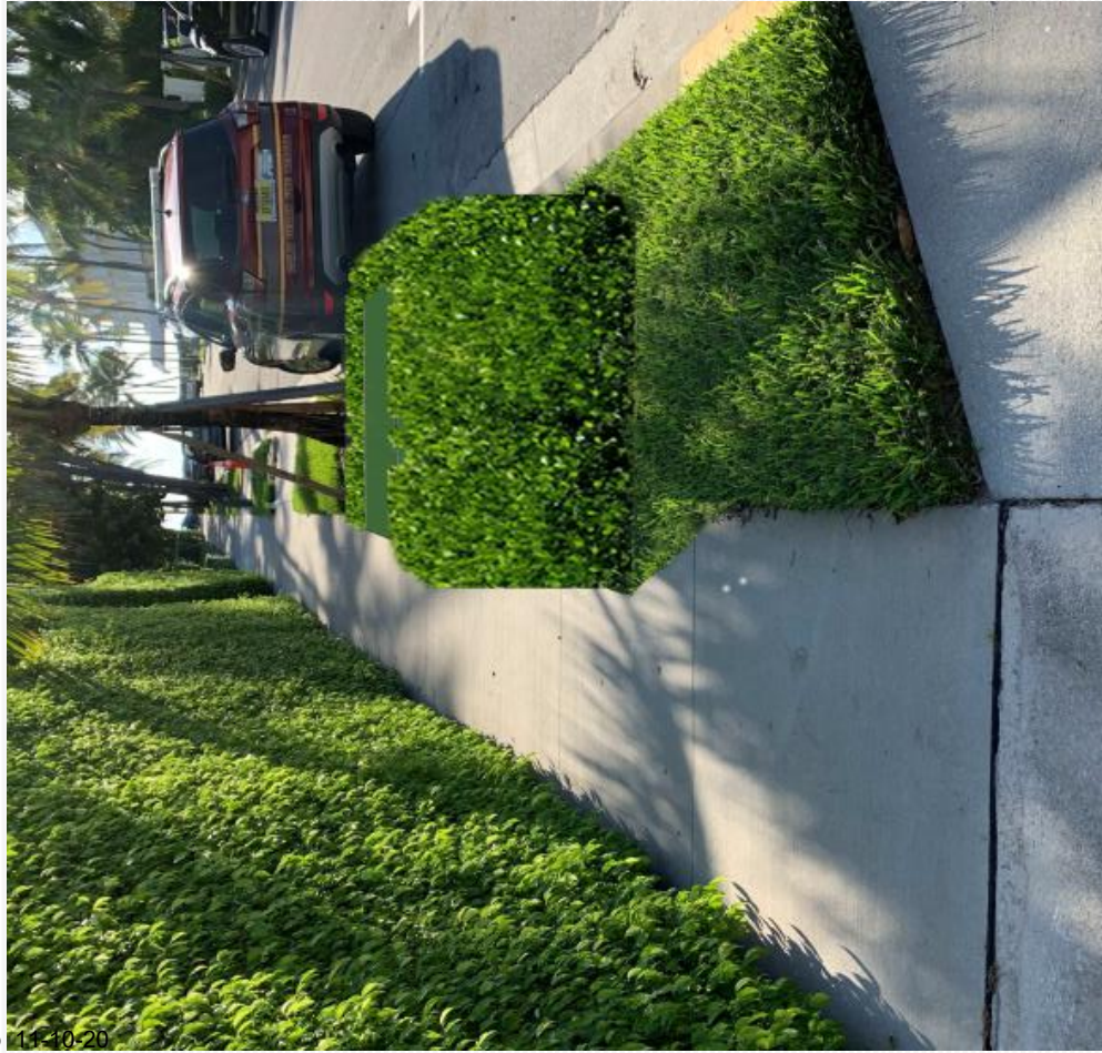
Typical Transformer with Landscaping
