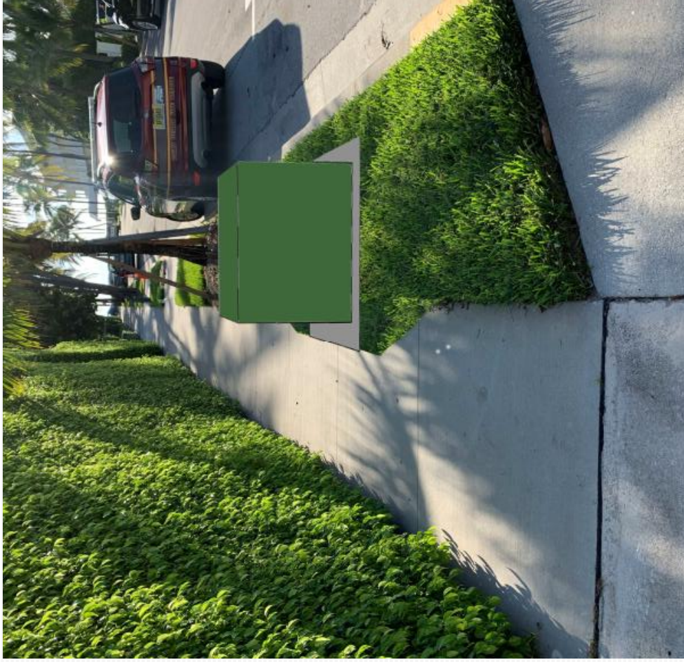
Typical Transformer without Landscaping
