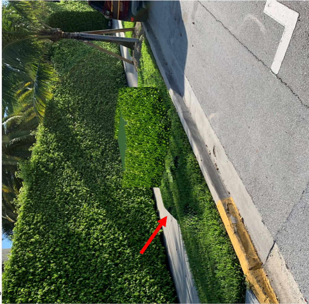
Typical Transformer with Landscaping
