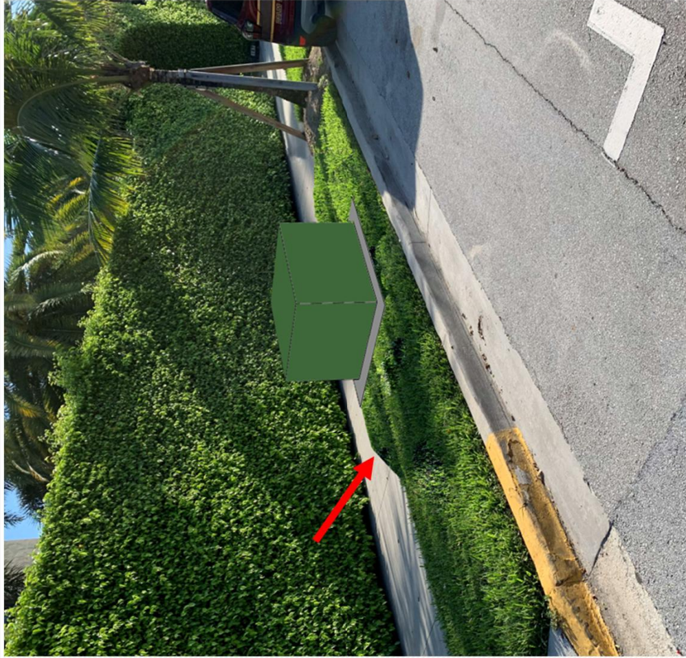
Typical Transformer without Landscaping
