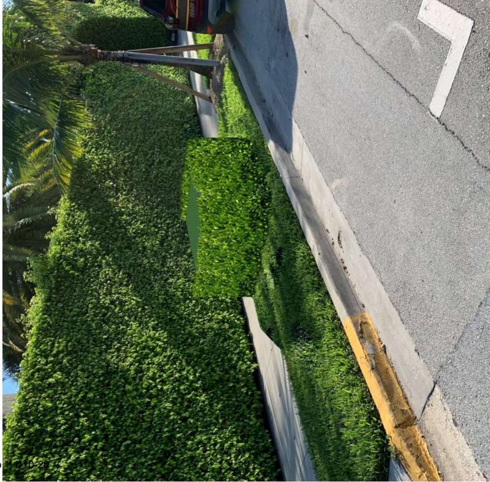
Typical Transformer with Landscaping
