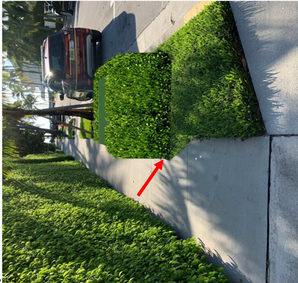
Typical Transformer with Landscaping
