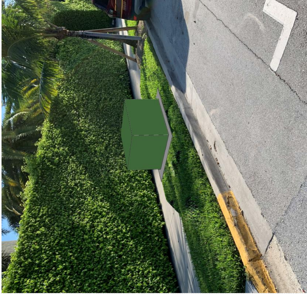
Typical Transformer without Landscaping
