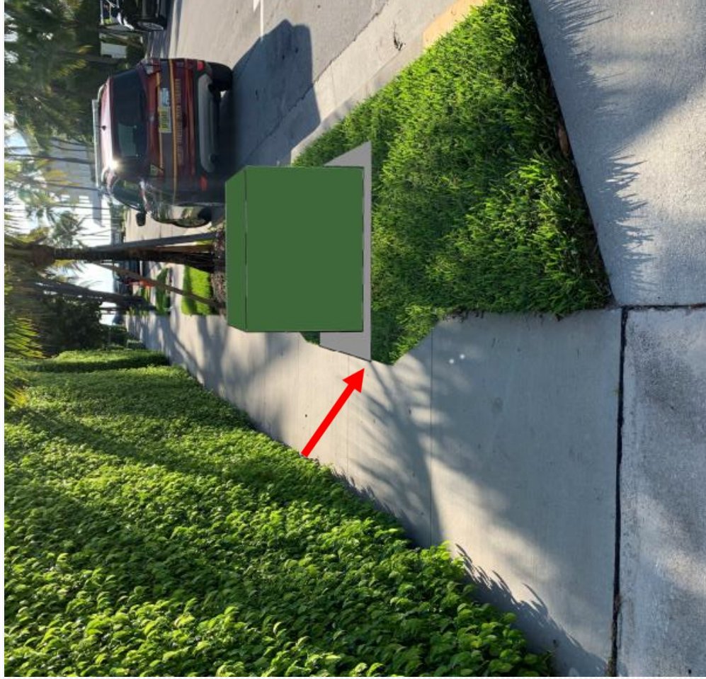
Typical Transformer without Landscaping
