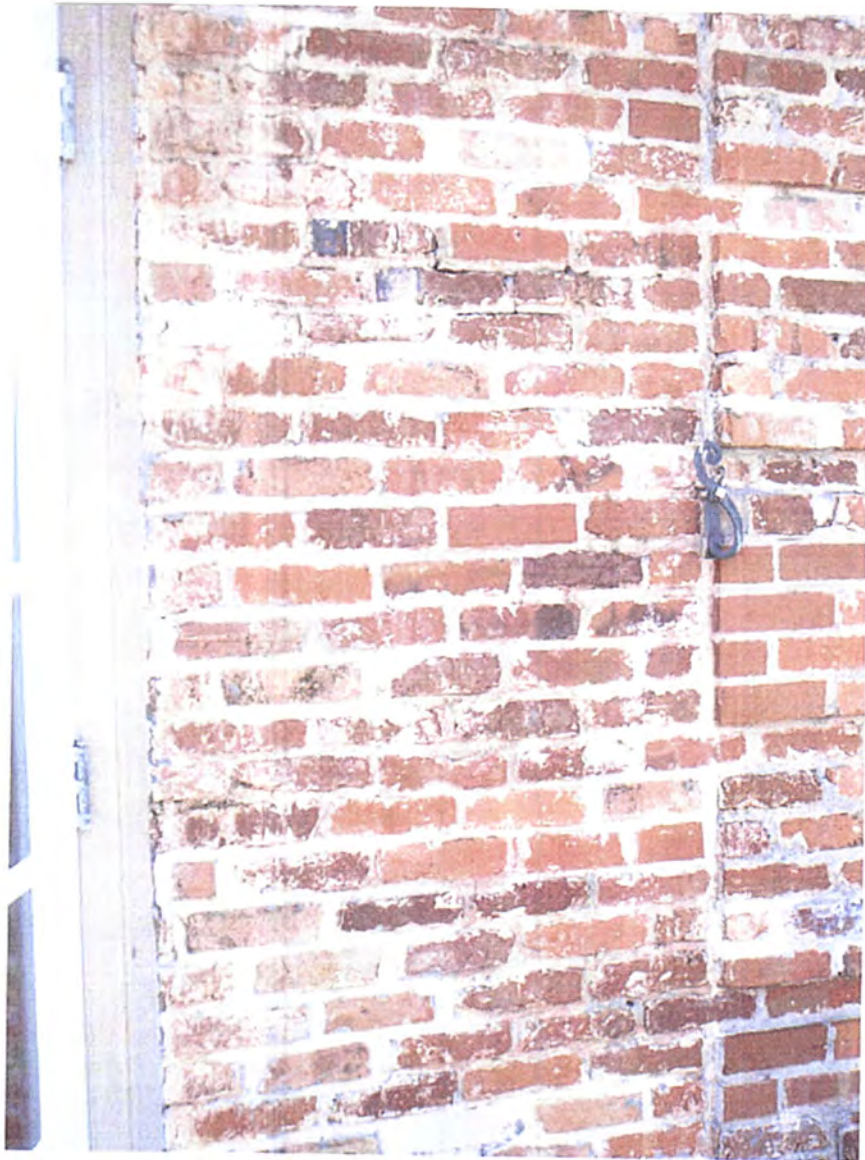
Sample of Brick Deterioration near Bay Window
