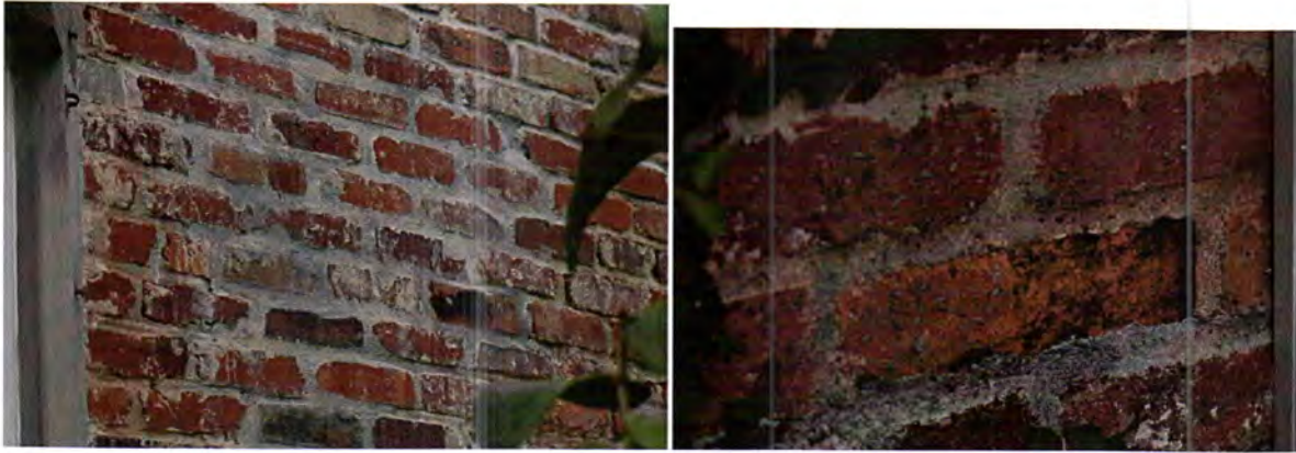
Fig. 17, The masonry is laid in running bond and has been repointed with hard (Portland Cement) mortar instead of a soft lime mortar, which is destructive and has caused spall in the under-fired used brick.
