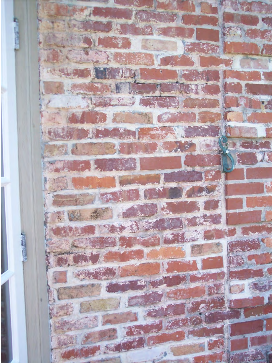
Sample of Brick Deterioration near Bay Window
