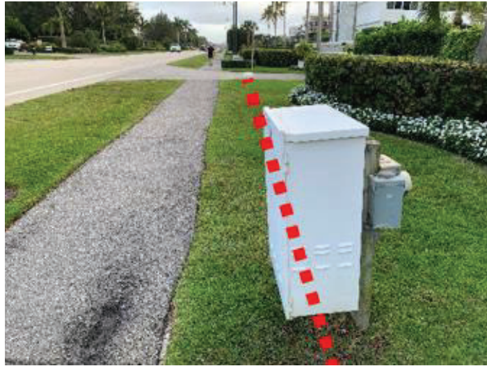
Existing Communications Utility Panel
