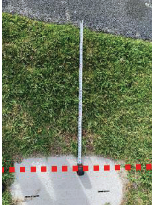
Existing Communication Pullbox
