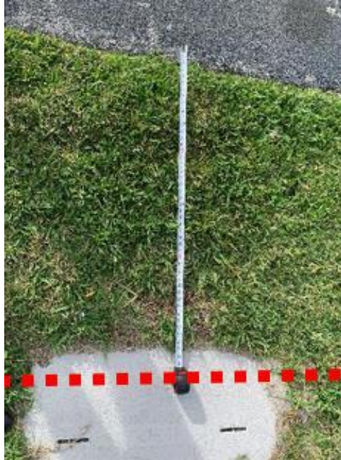
Existing Communication Pullbox
