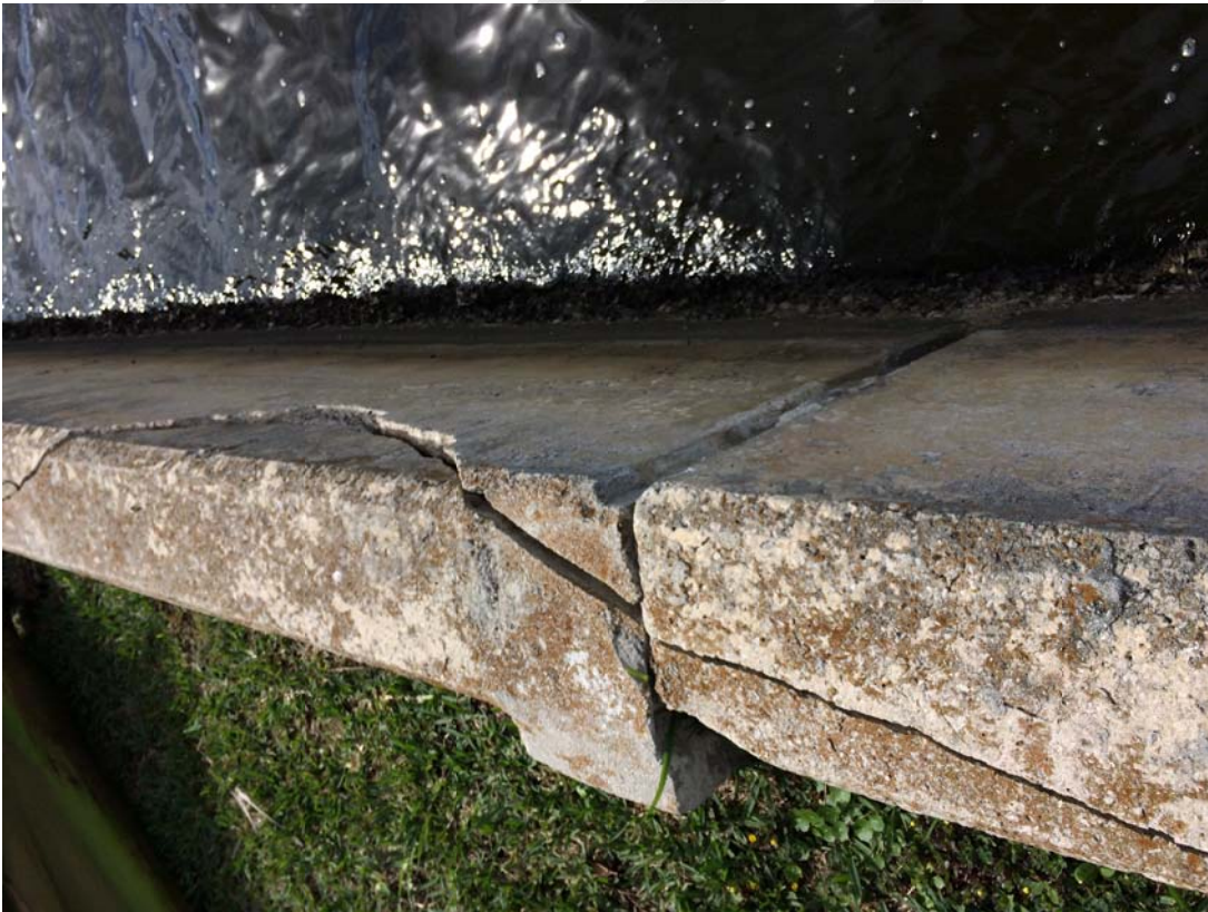
Figure 8.6: Cracking in the Bulkhead
