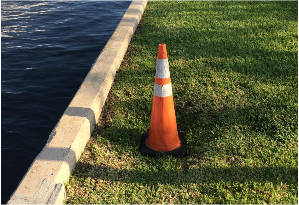
Figure 3.17: Sta 10+80. Area with backfill loss.
