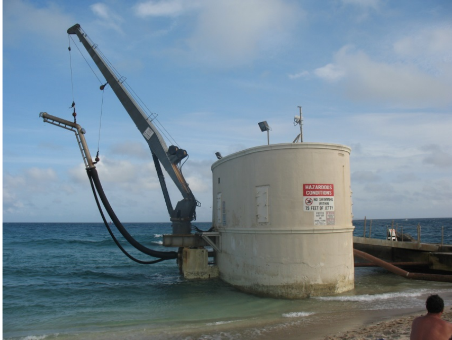
Figure 1. Lake Worth Inlet sand transfer plant (STP) north of the inlet.
